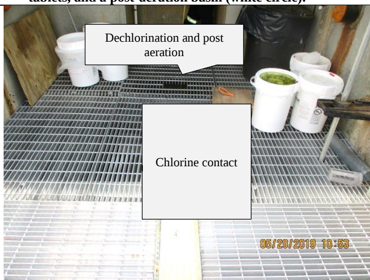
6. Looking from the location of photo 5 toward the chlorine contact, dechlorination and post-aeration areas.
