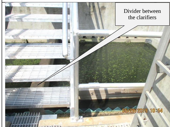
5. Two clarifiers at the base of the steps of the structure shown in photo 4.
