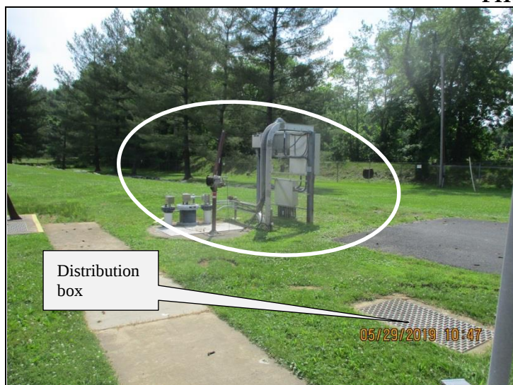
1. Influent pump station (white circle).
